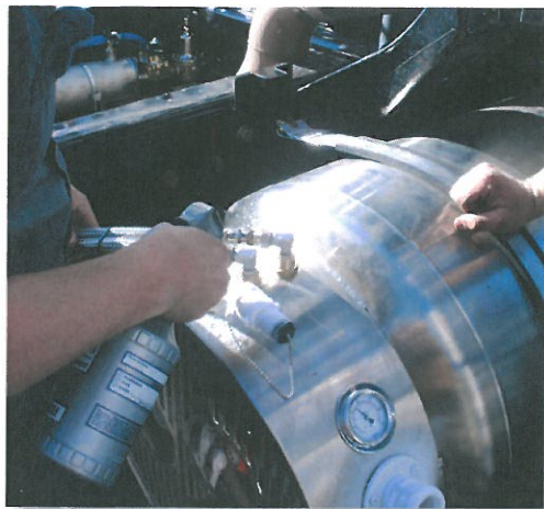
Dual-fuel systems can store gas in compressed or liquefied form. This is an LNG tank being installed by technicians at another WheelTime member, Smith Power in Salt Lake City.
